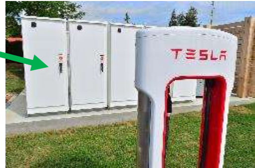
Mega-Watt EV Charging Station
