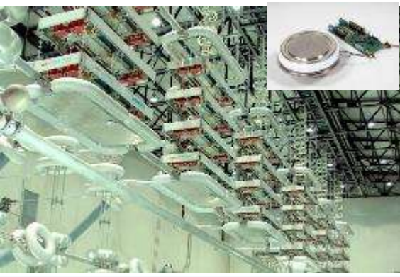
HVDC Thyristor Valve Building in China's 800 kV Power Station
